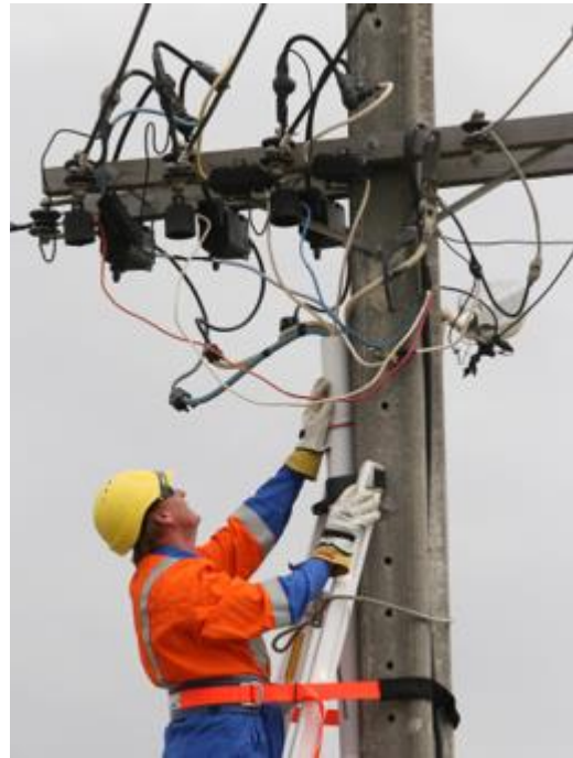
Pole Mounted Fuses
